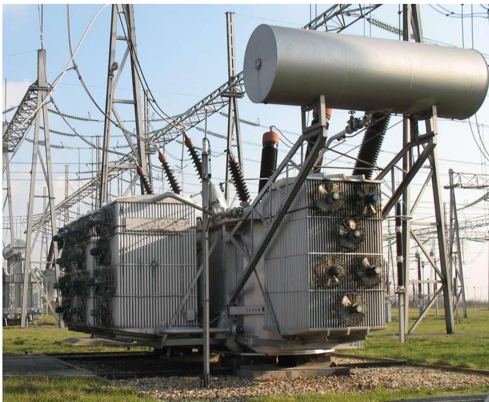
Figure 1 A transformer substation in the vicinity of the mine
