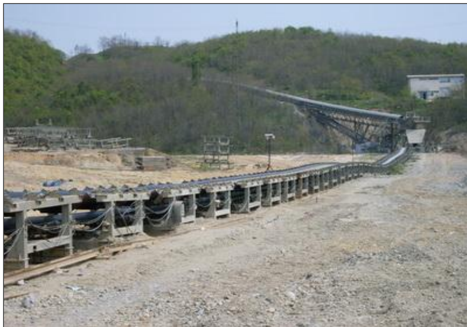
Figure 2 A part of a conveyor system for the transportation and disposal of tailings
