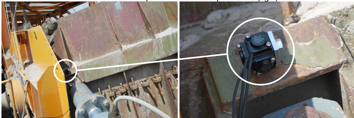
Figure 3 Vibration measurement – accelerometer placement on the hydraulic cylinder of the shield (left) and detail of 3D accelerometer Kistler K-Beam
